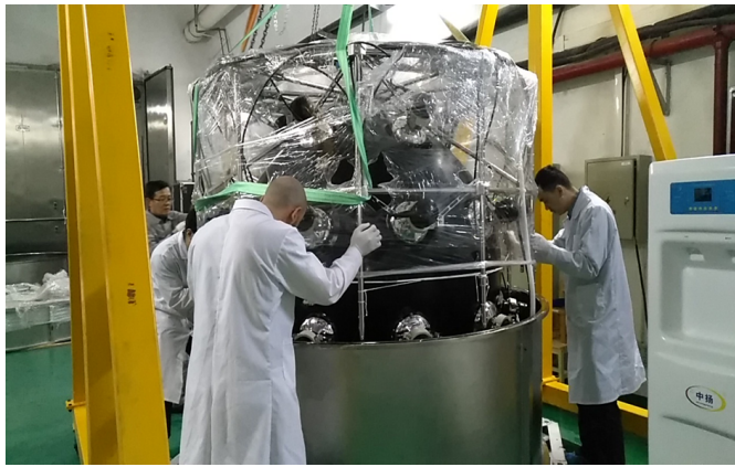
(c) Hoist the whole inner structure into the bottom part of the stainless steel tank.
